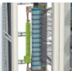
Connection on terminals and earth bar
