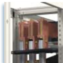
Horizontal busbar connection
